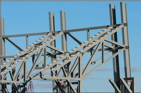
Figure 2 — The 14 inch by 6 inch high typical upper seating bowl prefabricated shippable raker trusses, which were designed to maximise shop assembly and simplify erection.
