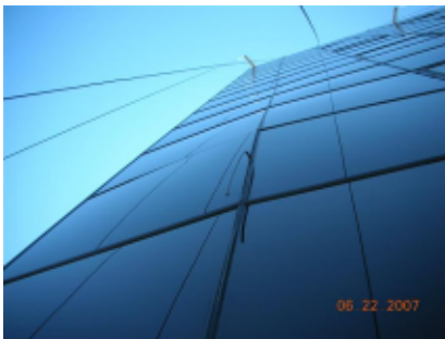
Bowed spandrel glass before repair
